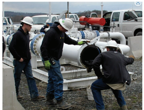
Figure 6. Technicians' proximity to pipeline traps.
