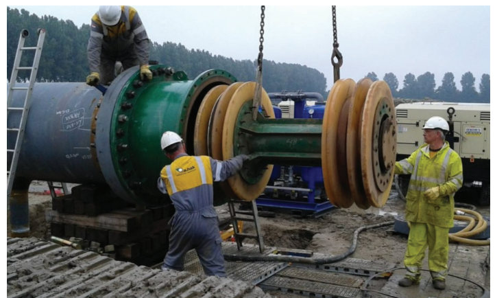
Figure 6. Technicians' proximity to pipeline traps.
